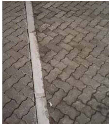
Photograph 1 – Anchor beam, showing gap due to creep of blocks immediately downside of anchor beam
