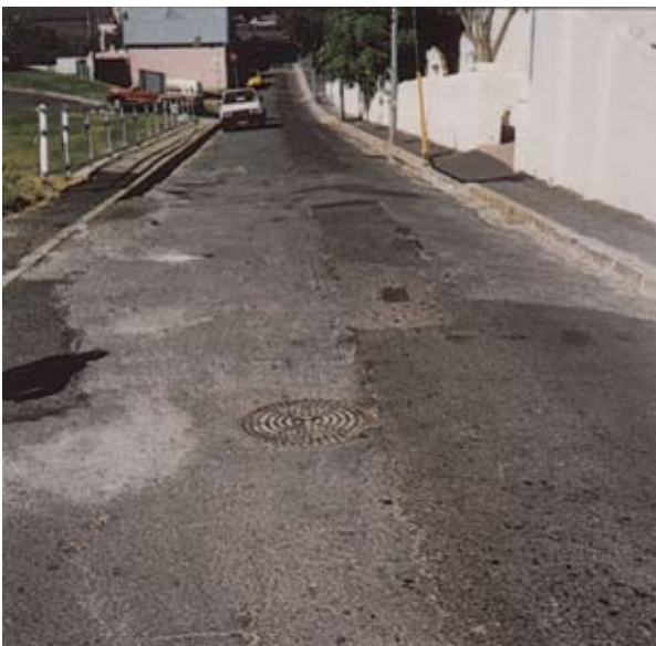
Photograph 8 – Upper Rhine Road - section still to be rehabilitated
